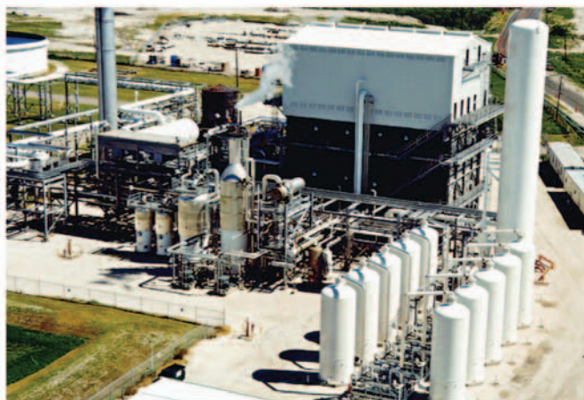
FIG. 1 Typical 50 million standard cubic ft/day H 2 plant.
