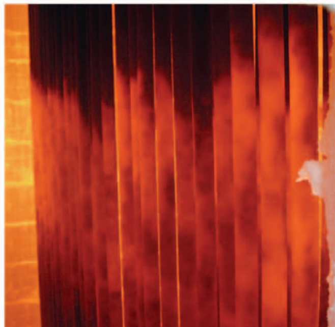
FIG. 3 Reformer tubes exhibiting the possible effects of carbon formation, sulfur poisoning, catalyst deactivation and/or catalyst attrition.
