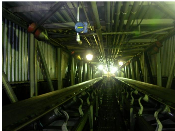
FIGURE 6: LOOKING DOWN THE MAIN CONVEYOR STRUCTURE. A CO MONITOR LOCATED ABOVE AND LEFT OF CENTER. TWO CONVEYOR BELTS ON EITHER SIDE, REDUNDANT TO MINIMIZE THE POTENTIAL OF SHUTTING DOWN THE PLANT IF A SINGLE CONVEYOR SHUTS DOWN.
