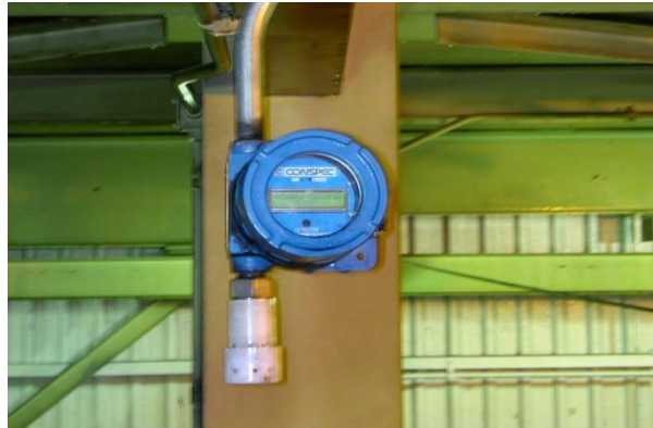
FIGURE 5: TYPICAL CO MONITOR INSTALLED ALONG A BELT HEAD DRIVE LOCATION. NOTE THE WHITE CAP ON THE SENSOR HEAD. THIS IS THE SPLASH GUARD USED TO PREVENT WASH-DOWN WORK FROM LOADING THE SENSOR WITH WATER.
