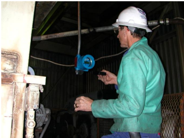
FIGURE 4: A CO MONITOR UNDERGOING CALIBRATION DURING INITIAL INSTALLATION AT THE TOP OF THE CONVEYOR STRUCTURE.
