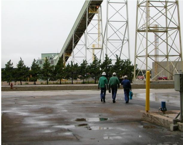
FIGURE 3: THE MAIN CONVEYOR STRUCTURE AT HARRINGTON RISES FROM THE CRUSHER BUILDING BEHIND THE TREES. THE LIVE PILE, CAR DUMP, AND RECLAIM TUNNEL ARE LOCATED ON THE FAR SIDE OF THE CRUSHER BUILDING. THE WALLS AND FLOORS ARE CORRUGATED METAL AND THERE ARE NUMEROUS OPENINGS IN THE STRUCTURE.
