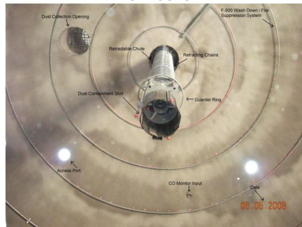
FIGURE 13: THE INSIDE OF A DOME SHOWING THE VARIOUS COMPONENTS AND THEIR PURPOSES.
