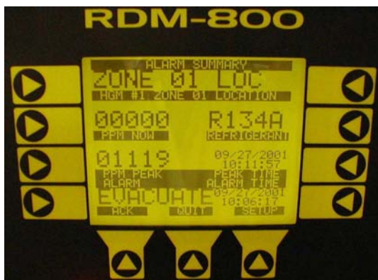
Alarm Detail Screen
